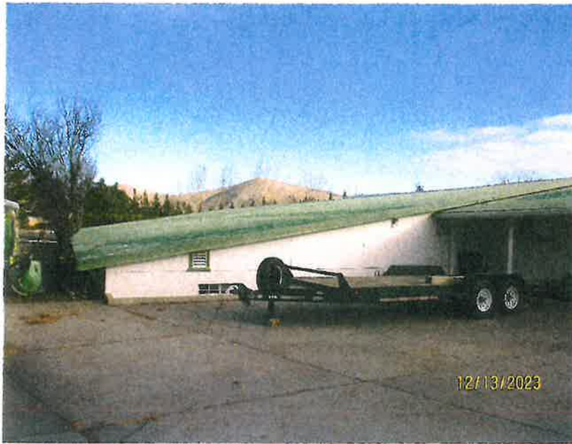
Exterior (accessibility issues – construction of building below grade)
