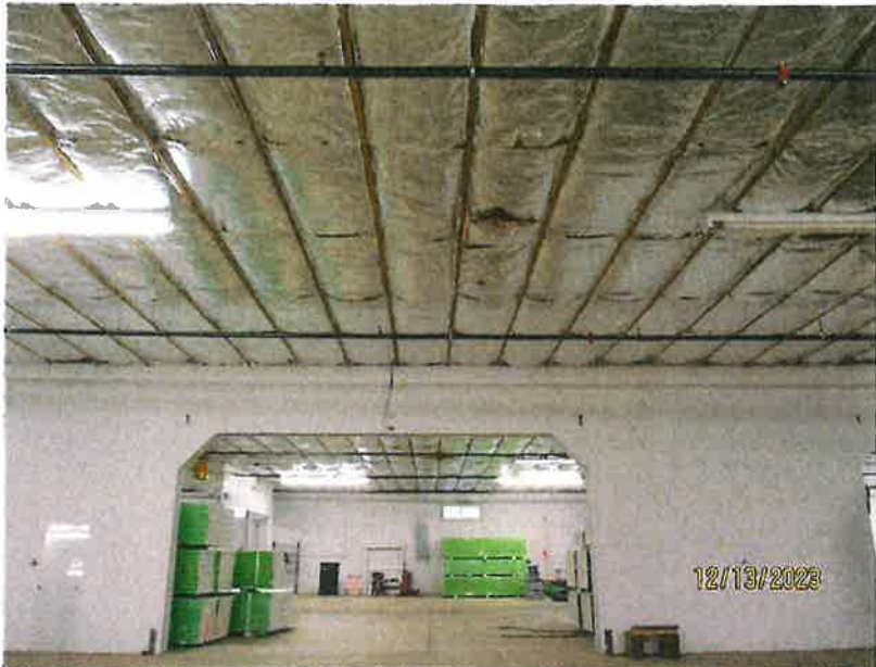
Interior water damage (insulation and walls)
